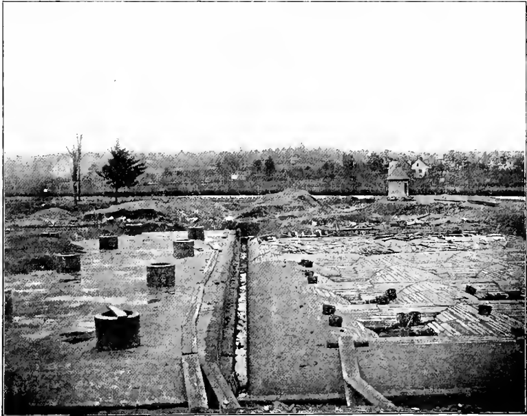
COVERED FILTER IN COURSE OF CONSTRUCTION, SHOWING WOODEN CENTERS FOR MASONRY VAULTING, SOMERSWORTH, N. H.
